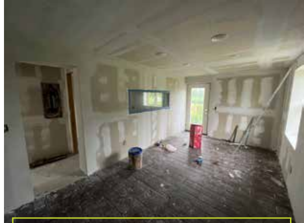
A former dairy farm's milking house being transformed into our station's office.
